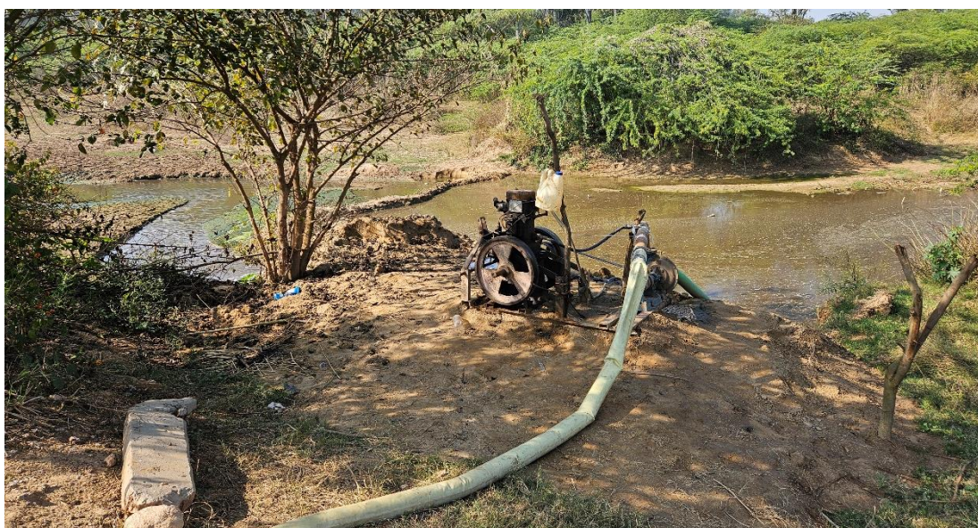
Figure 12: A farmer lifting water from the damaged check dam in Kheri Gujjar
